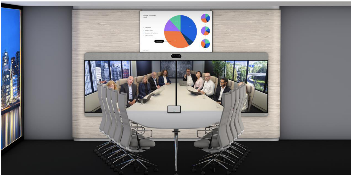
Figure 2. Point-to-point meeting in a large conference room
